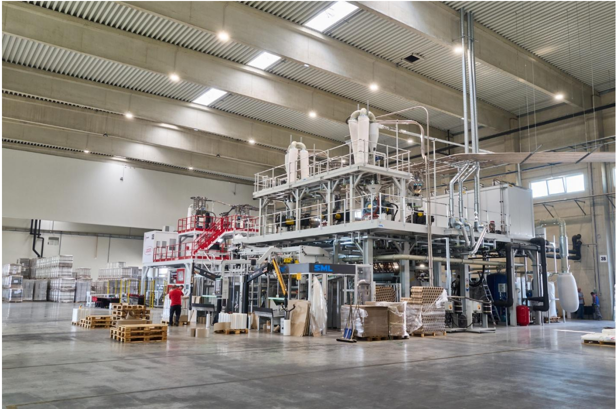
Figure 3 - Newly installed production lines in 2024.
