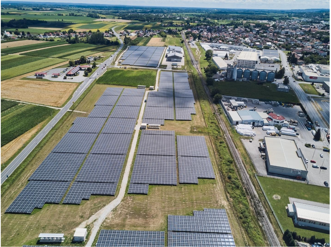
Figure 2 - Part of Bomark Pak's 15MW solar powerplant
